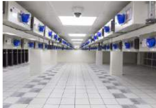
Data Center Development
