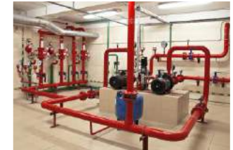
Plumbing and Sanitary Engineering
